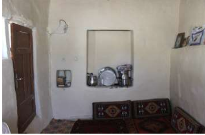
Foto 21. Birinci kat oda güney cephe (Photo 21. First floor the room south front)
