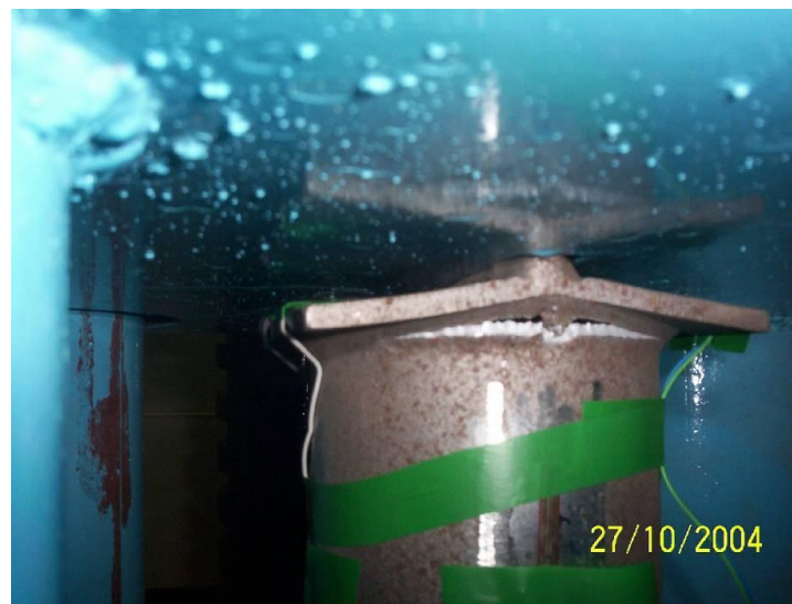
Figure 7. Weld fracture (114.6x6.3 CHS tube) (Figure 7. Fature de soudure (114.6x6.3 tube))
